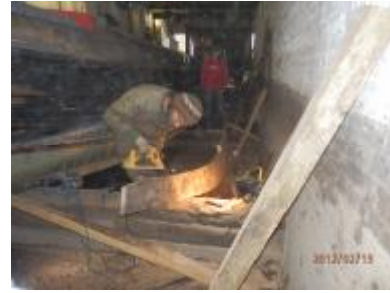
New flashes being prepared
